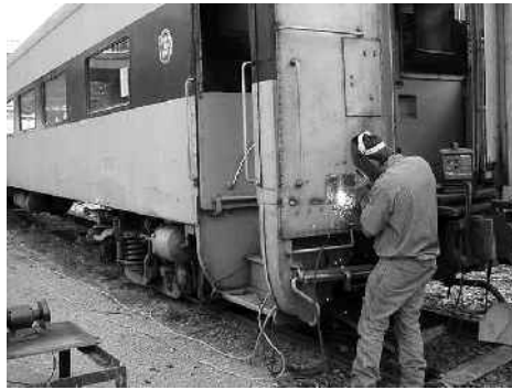
1318's end receives some welding repairs at Ozark Mountain Railcar. (John Suscheck photo)
