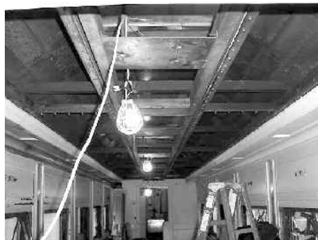
The ceiling of the 741 is seen after removal for clerestory inspection. (John Suscheck photo)
